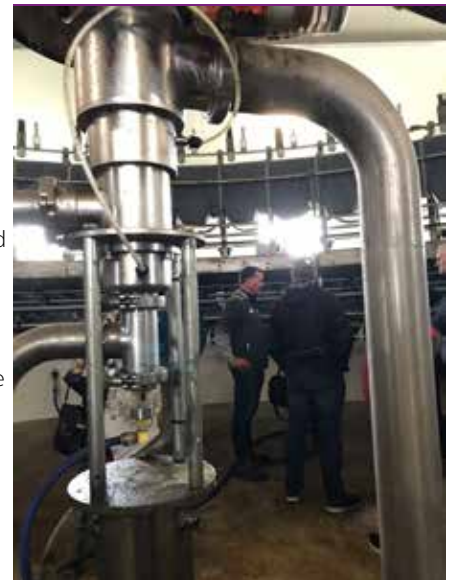
Equipment at Stewart Dairylands
